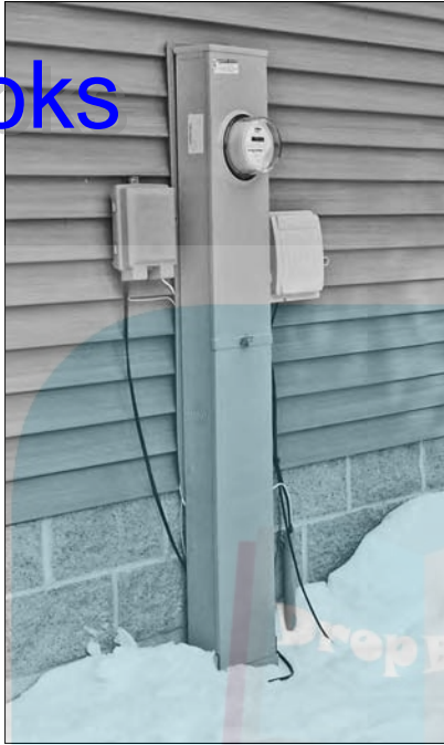
Figure 6-3: These sloppy cable TV and phone installations are susceptible to damage.
